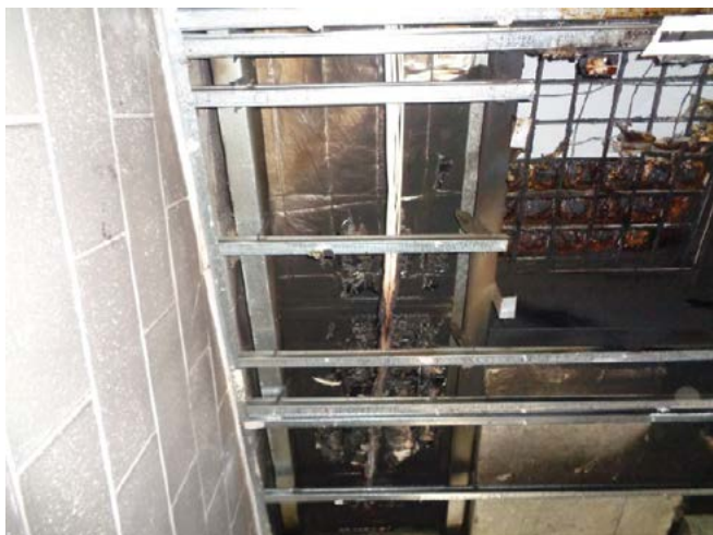
Photo 2: Ceiling and melted skylight in the foyer
