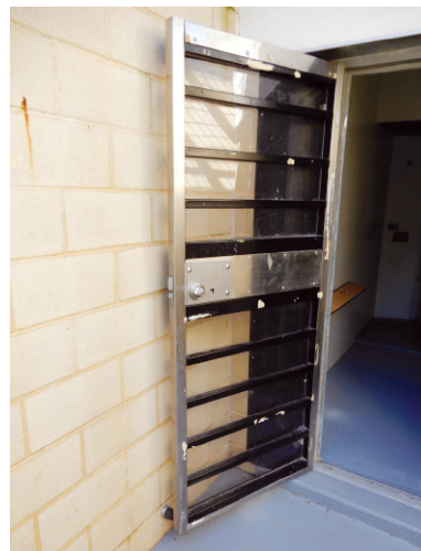
Source: Pedavoli Architects 'Management Unit Review' draft report. Door in ajar position but not locked to the wall.
